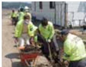
Recovering Lifeline( infrastructure)
